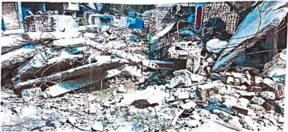
Fig. 3 Debris at Site (photo taken on 10.10.2023)
