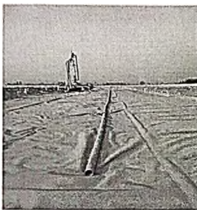
Perforated Pipes at RMS Area
